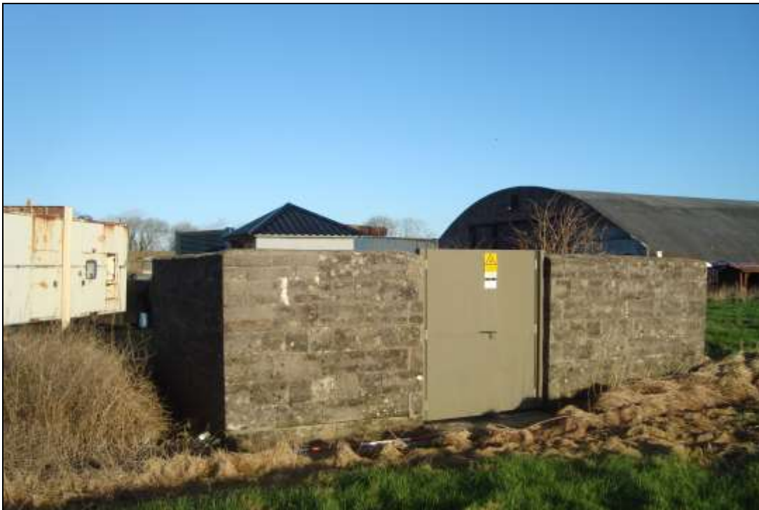
Plate 58: Modern wall surrounding the transformer kiosk
