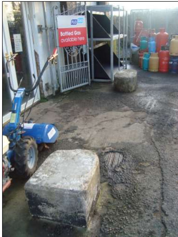
Plate 80: Concrete hurters in front of the bay entrances
