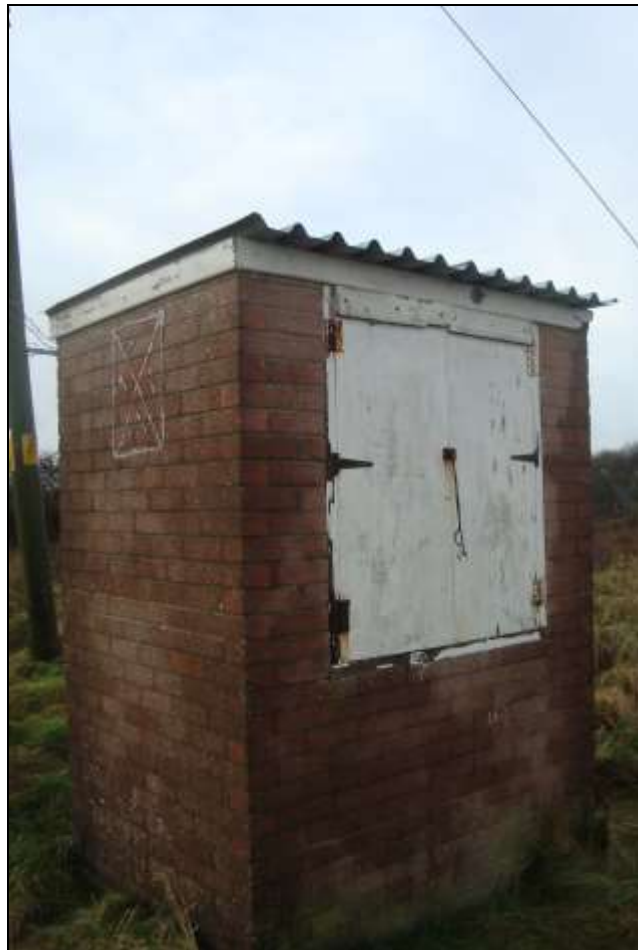
Plate 32: Modern transformer kiosk stands were the original once stood
